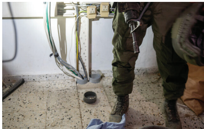
Electrical cables found by the IDF that lead directly from UNRWA’s main Gaza headquarters into an underground Hamas data centre located beneath it (Image: IDF)
